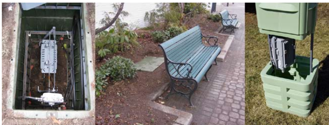
Figure 5. BelAir 100S vault and pedestal installations.
